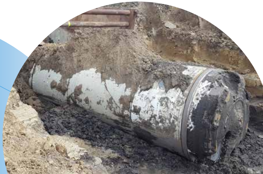
An Earth Pressure Balance Machine (EPBM) exits the Cliff Avenue crossing in Sioux Falls, South Dakota.
