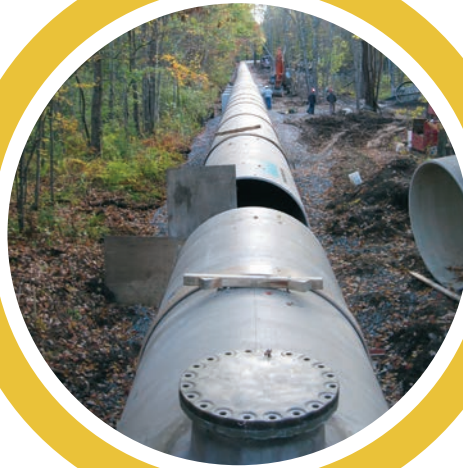
84-inch diameter Hydro-Electric Penstock in New Hampshire
